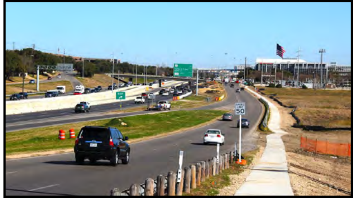
Sidewalk construction along northbound MoPac frontage road at Anderson Lane. Photo from MoPac Improvement Project website
